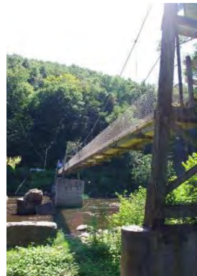
Hendricks Swinging Bridge, a unique experience
